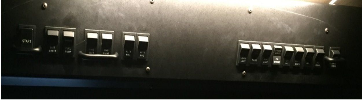
Image 16: Overhead Switch Panel
