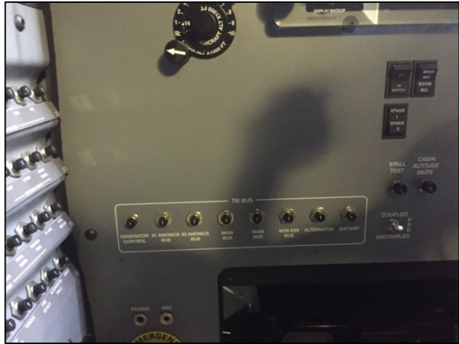
Image 11: Pilot Switches (Lower Left)
