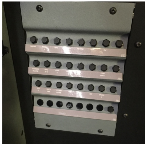
Image 15: Co-Pilot Circuit Breaker Panel
