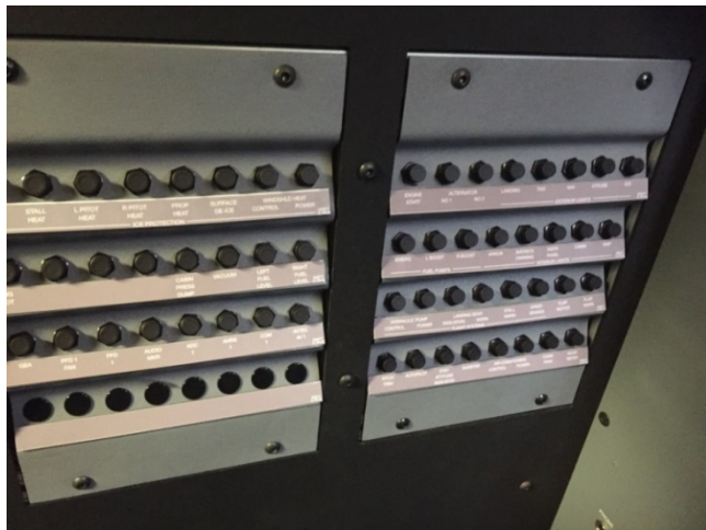
Image 14: Pilot Circuit Breaker Panel
